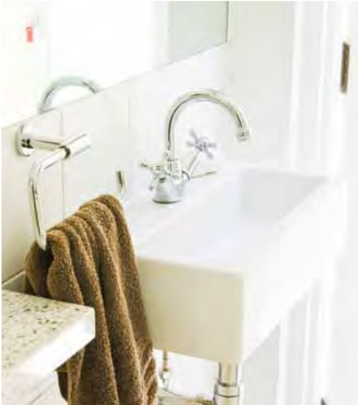
⤵ The downstairs toilet/laundry, coming in at a mere 3.78m², defies its dimensions with a large mirror and white, light-reflecting surfaces. It has taps for a tight fit: Bastow Georgian basin mixer twinner with an Ostar 9045 wall-mounted basin. Mixers with separate hot and cold taps are more energy-efficient than single levers, which tend to be left in the middle position.
